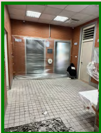
廁所地板整修前
